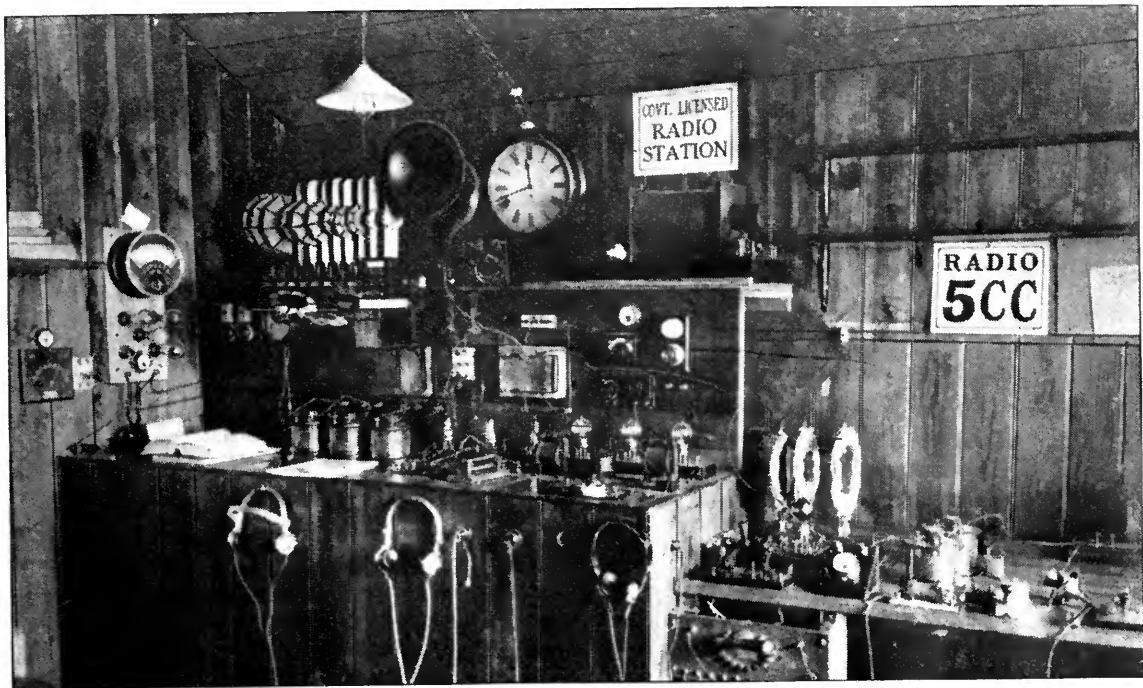
A GOOD ENGLISH AMATEUR RADIO INSTALLATION Is this station 5CC at Bath
